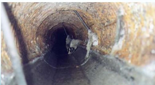
18 " Dia. RCP Sanitary Interceptor With Wall Deterioration
