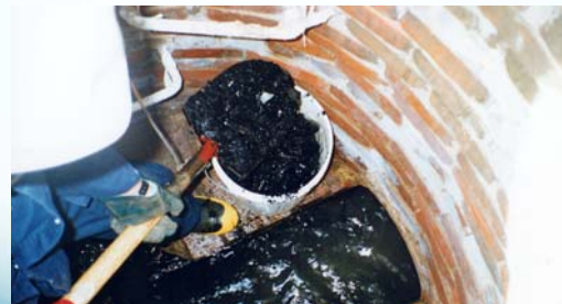
Obstructed 12" Dia. VCP
