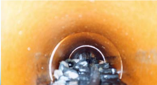
12" Dia. VCP Parallel Relief Sewer Obstructed by Intruding Utility Pole, Rocks & Sediment
