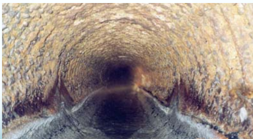
18 " Dia. RCP Sanitary Interceptor With Wall Deterioration
