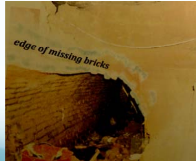
20 ft long by 7 ft. wide Void // to deteriorating brick sewer
